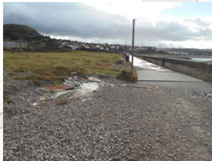
Repair base layer and overlay with tarmac surface. Add edge protection as required
