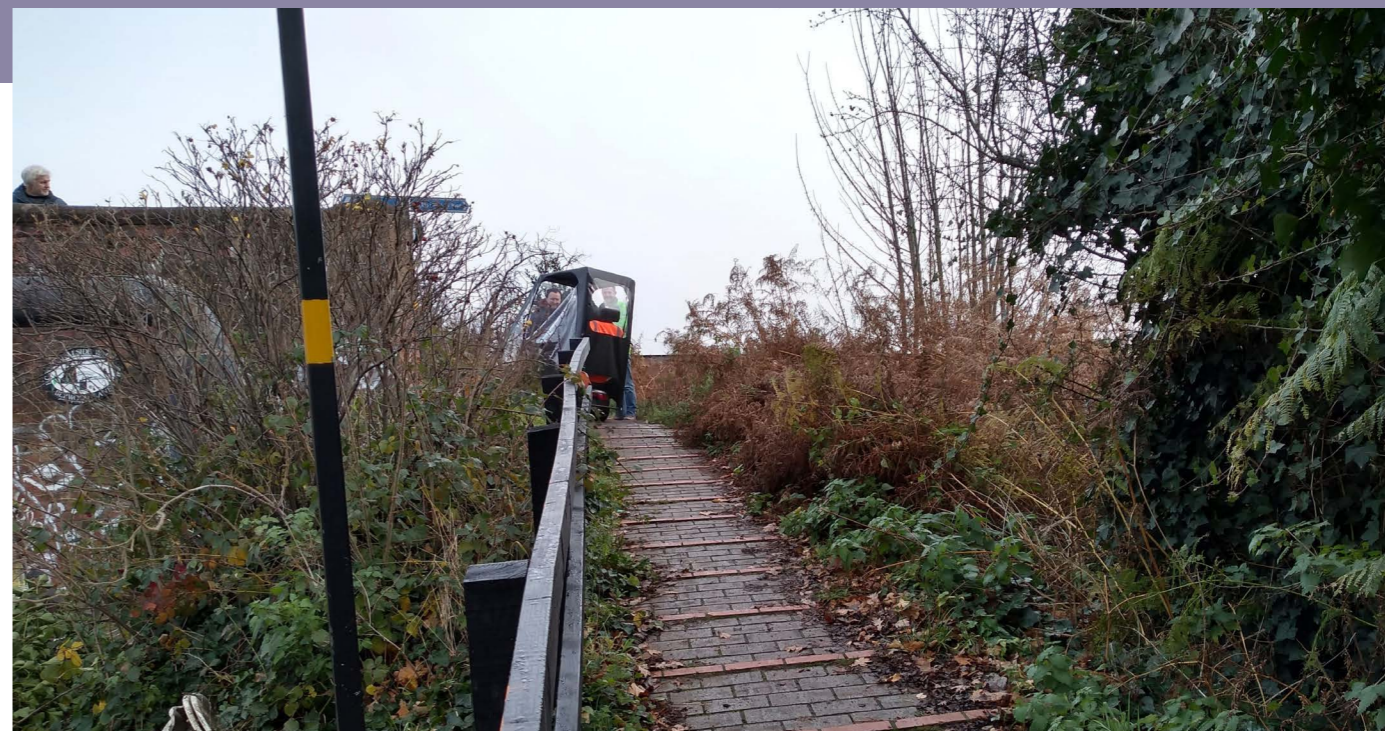
Fig 27. Overgrown vegetation on canal access in Tyburn area. Image Credit: Sustrans
