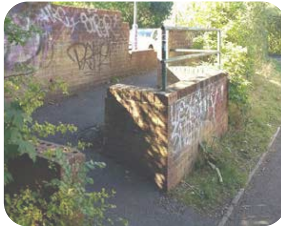
The existing Rose Green Road access is of poor quality, and restricts access to many users due to the tight angles and steep gradient.
