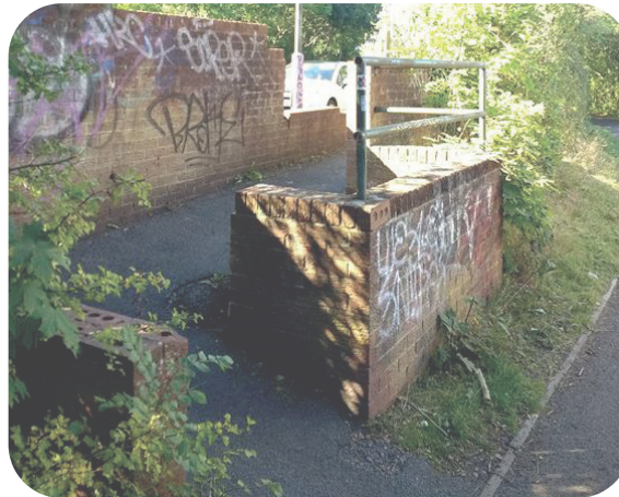
The existing Rose Green Road access is of poor quality, and restricts access to many users due to the tight angles and steep gradient.
